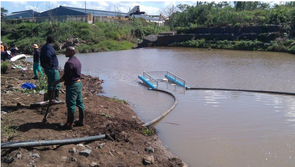
90mm HDPE pipes were used as the flotation guides which were capped at the ends.
